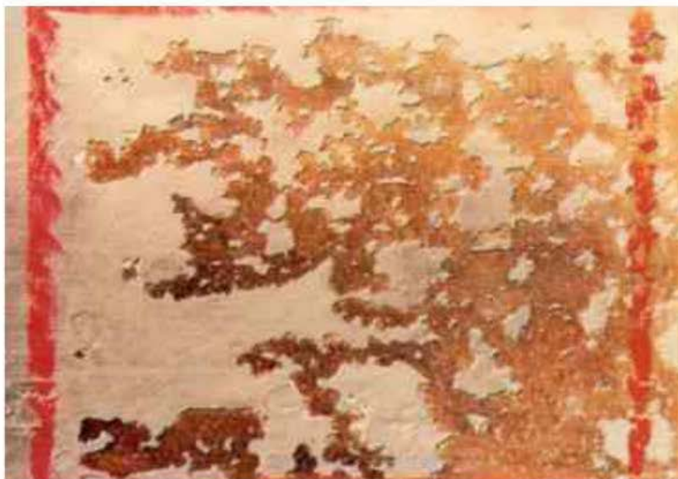
b) section from Figure 12 a): clear illustration of the defect at increased magnification
